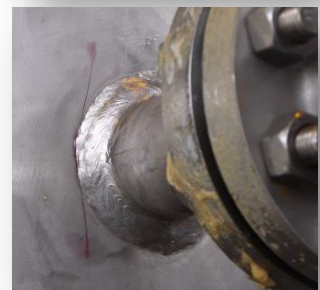
Figure 2: Piping failure examples
