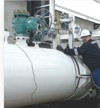
Figure 5: Piping Vibration Assessment (including small bore piping during normal and transient operations)
