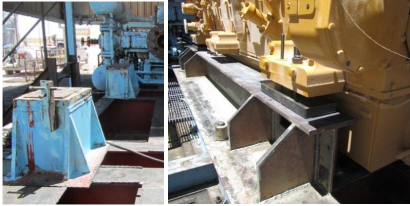
Figure 5. Existing engine pedestals (left) and new engine rails (right)
