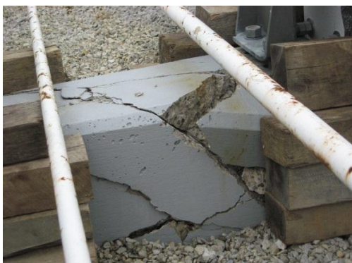
Figure 2. Examples of pipe clamp damaged by incorrect piping analysis
